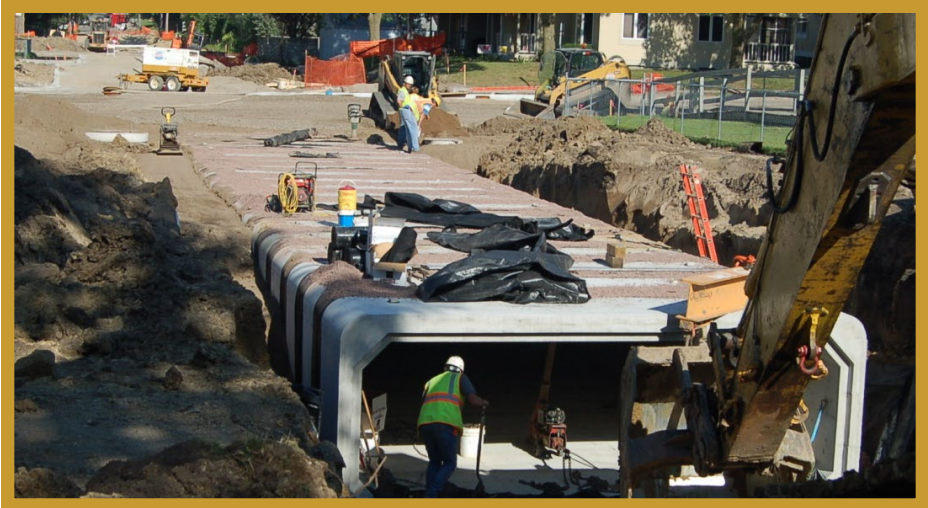
Underground Storage & Treatment
