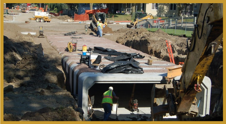
Underground Storage & Treatment
