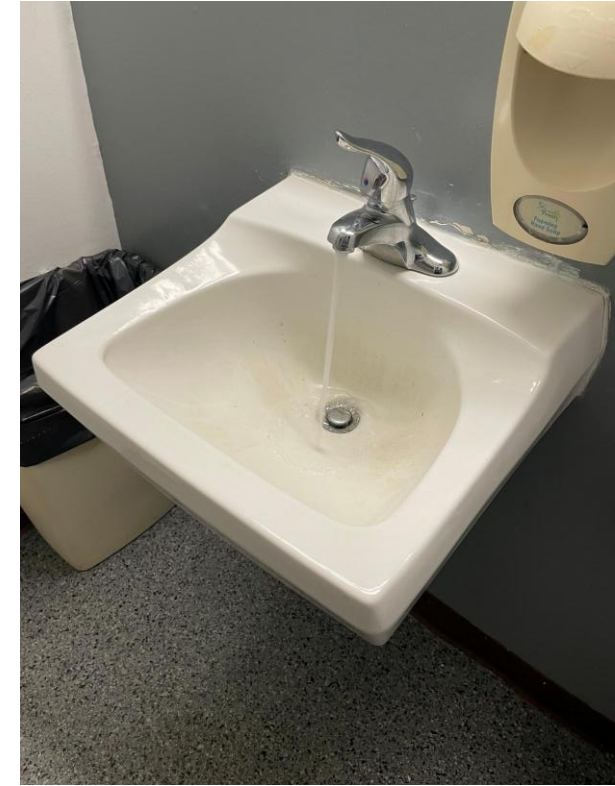
Old Plumbing fixtures contributing to water waste: targeted for replacement with low-flow models.
