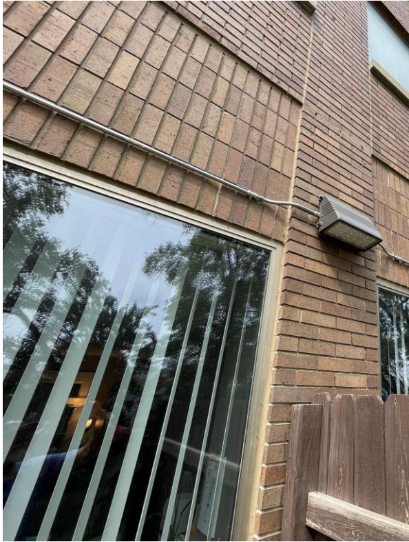
Inefficient exterior lighting to be replaced with LED fixtures to increase energy savings.
