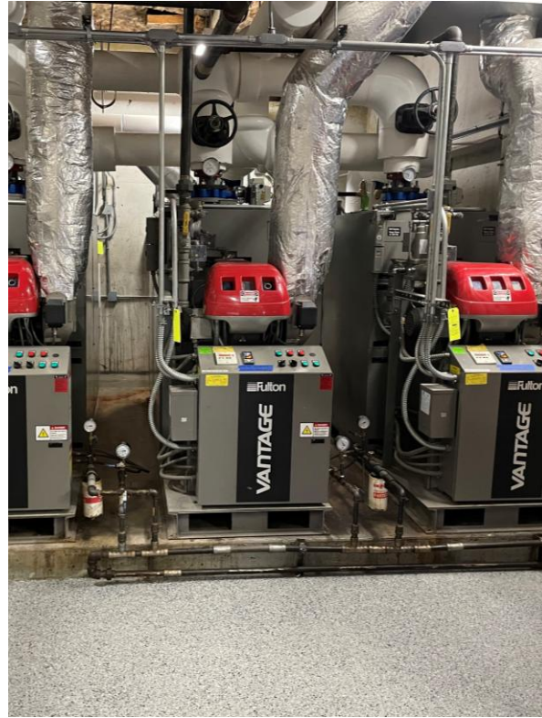
Existing boiler system to be upgraded to a high-efficiency model to qualify for RRI.
